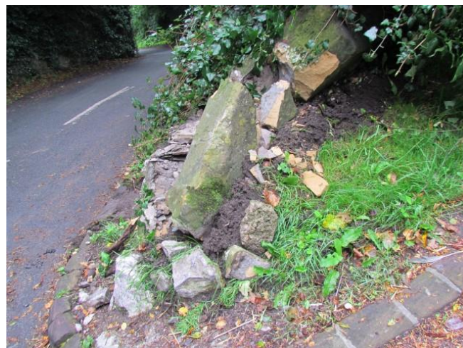
The damaged milestone at the top of The Slough
